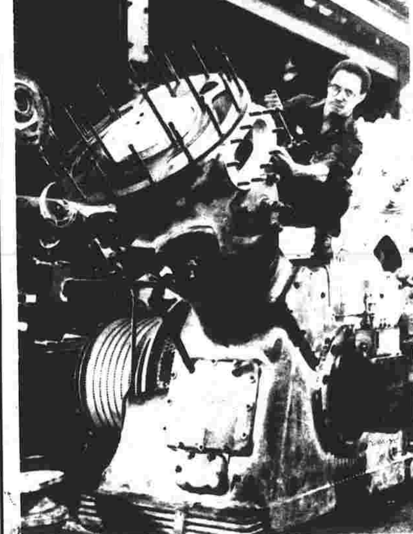
Edwin Alvarez isn't creating some metallic monster for an out space epic, but reassembling a 2,000 horsepower reciprocating air compressor for remanufacturing at General Electric American Air Compressor Services shop in North Bergen, N.J. The GE facility specializes in servicing and rebuilding reciprocating air compressors for such industries as glass, petrochemicals and oil refining. (UPI photo)
